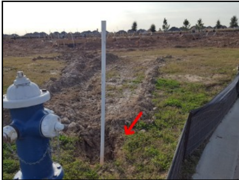
Water meter location at front left corner
