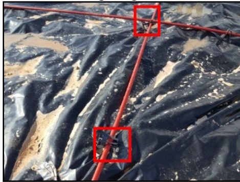
Cable chairs not properly seated
