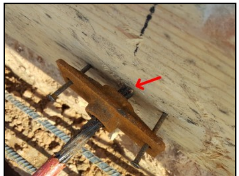
Cable in contact with form at rear right elevation
