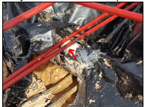
Cables in contact with drain at rear elevation
