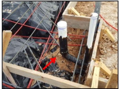
Evidence of cave-in at right elevation
