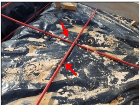
Cables not raised off pad
