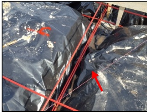
Evidence of cave-in at rear elevation
