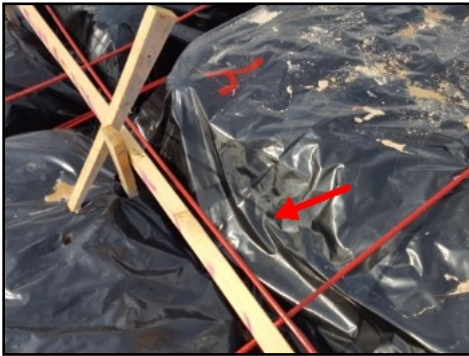
Evidence of cave-in at rear elevation
