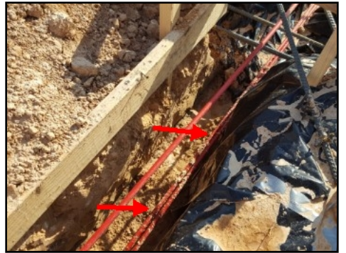
Cables not raised off beam
