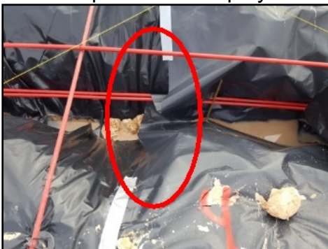
Poly not sealed/secure in place
