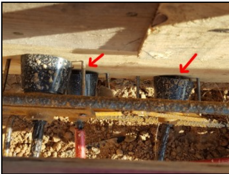
Pocket formers not flush to form at left elevation
