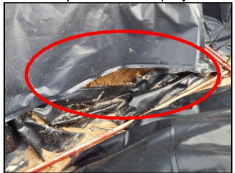
Poly not sealed/secure in place
