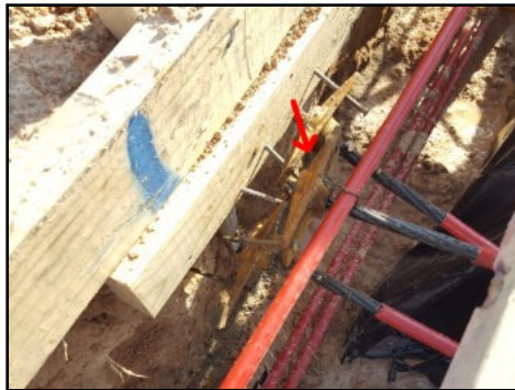
Cable not secure in place at garage
