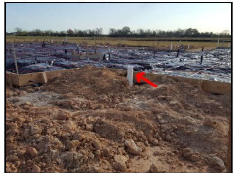
Main sewer clean out at front right elevation
