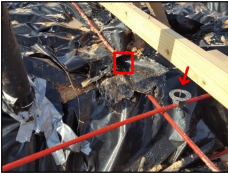
Cable chair not properly seated
