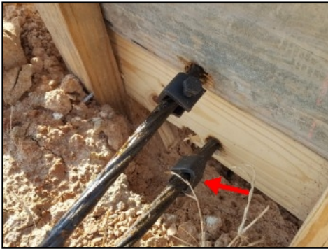
Cable clamp not secure in place
