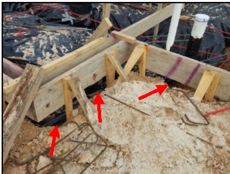
Void present at right elevation
