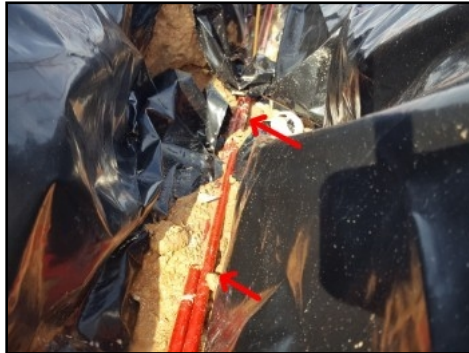
Cables not raised off beam
