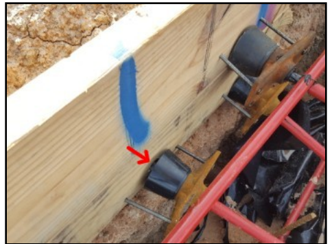
Pocket formers not flush to form at rear elevation
