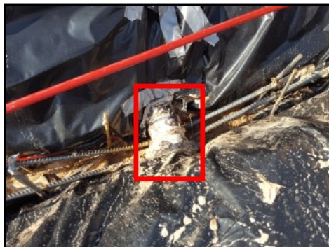
Drain line not coated with mastic
