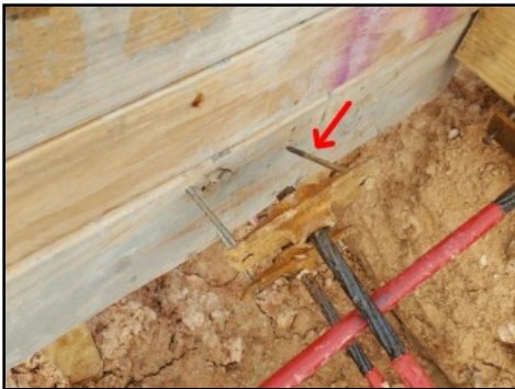
Cable not secure in place at front elevation
