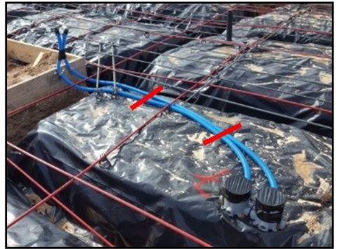
Conduit material not secure in place
