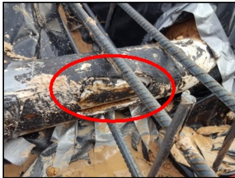
Damaged drain line at left elevation
