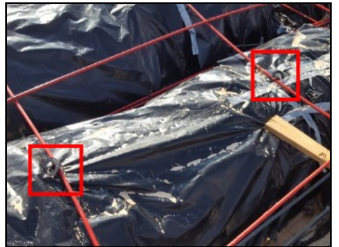
Cable chair not properly seated
