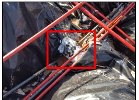
Drain line not coated with mastic
