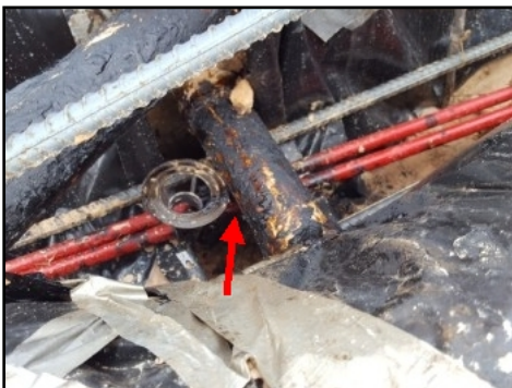
Cables in contact with drain at right elevation
