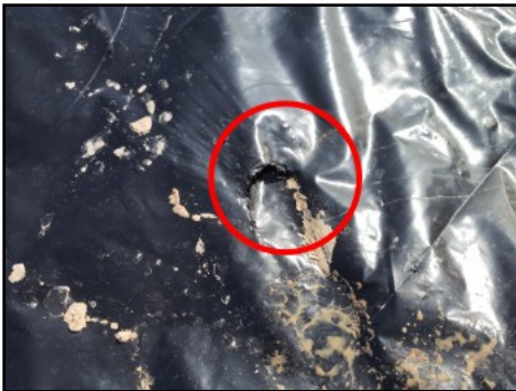
Repair torn/damaged poly
