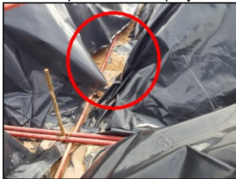
Poly not sealed/secure in place
