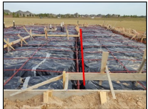
Missing cable at rear elevation
