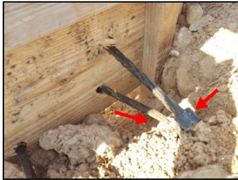
Cable clamps not secure in place
