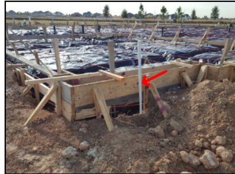
Main water line entry to home
