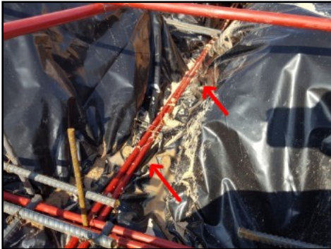
Cables not raised off beam at left elevation
